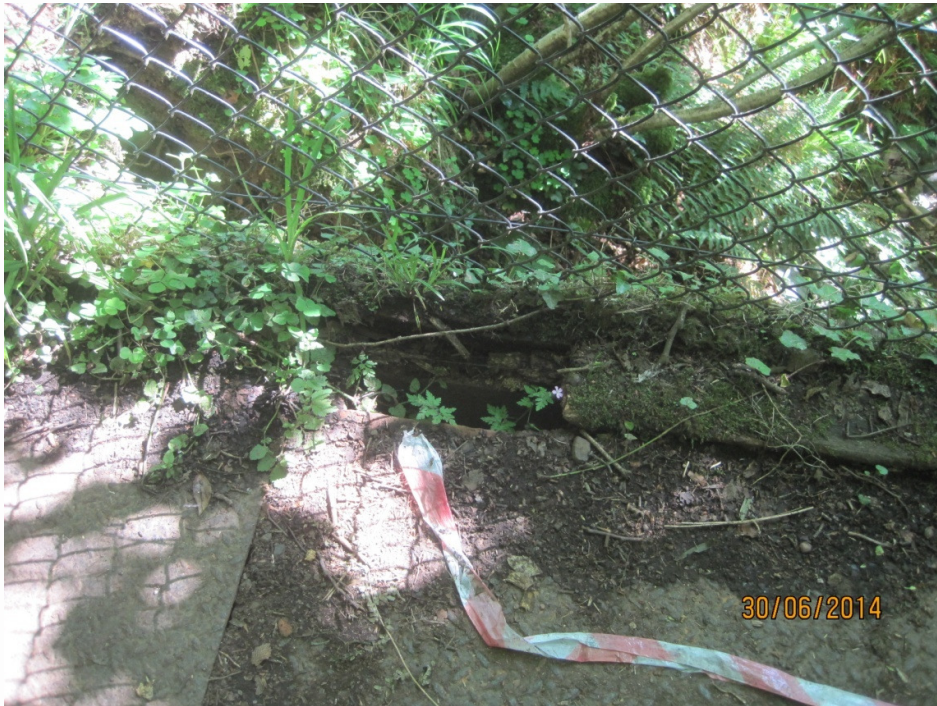
Figure 1 Rotting Deck Timber
